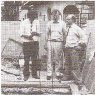
Professional Team. Surveying the start of Pile Pit no 2, Structural Engineer (Hockley & Dawson), Architect (Whitfield Partners), Site Engineer (Taylor Woodrow Construction Ltd).
