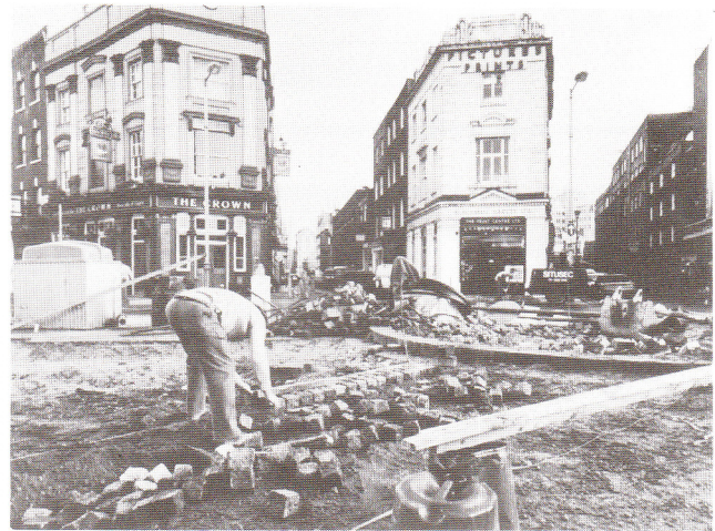
Reparing Seven Dials. Camden Council, with D.O.E. support, completely re-surfaced the Dials with pavoirs, cobbles and bollards, and created a central island in preparation for the reconstruction of the Sundial Pillar. This was part of an extensive programme of environmental improvements around Seven Dials which has involved tree-planting, pavement widening and traffic management.
