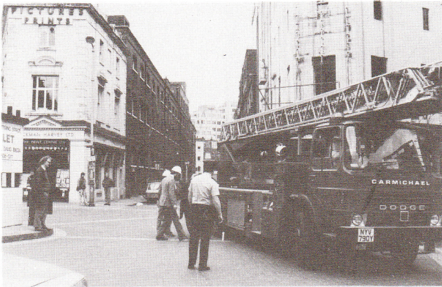
Borrowing a Fire Engine. To ensure that the foundation works could be carried out with minimal traffic disruption the Soho Firestation lent us their largest vehicle for an afternoon. It is pictured with representatives from the London Borough of Camden Planning and Works Department, the Metropolitan City Police, Whitfield Partners, Taylor Woodrow Construction Ltd etc.
